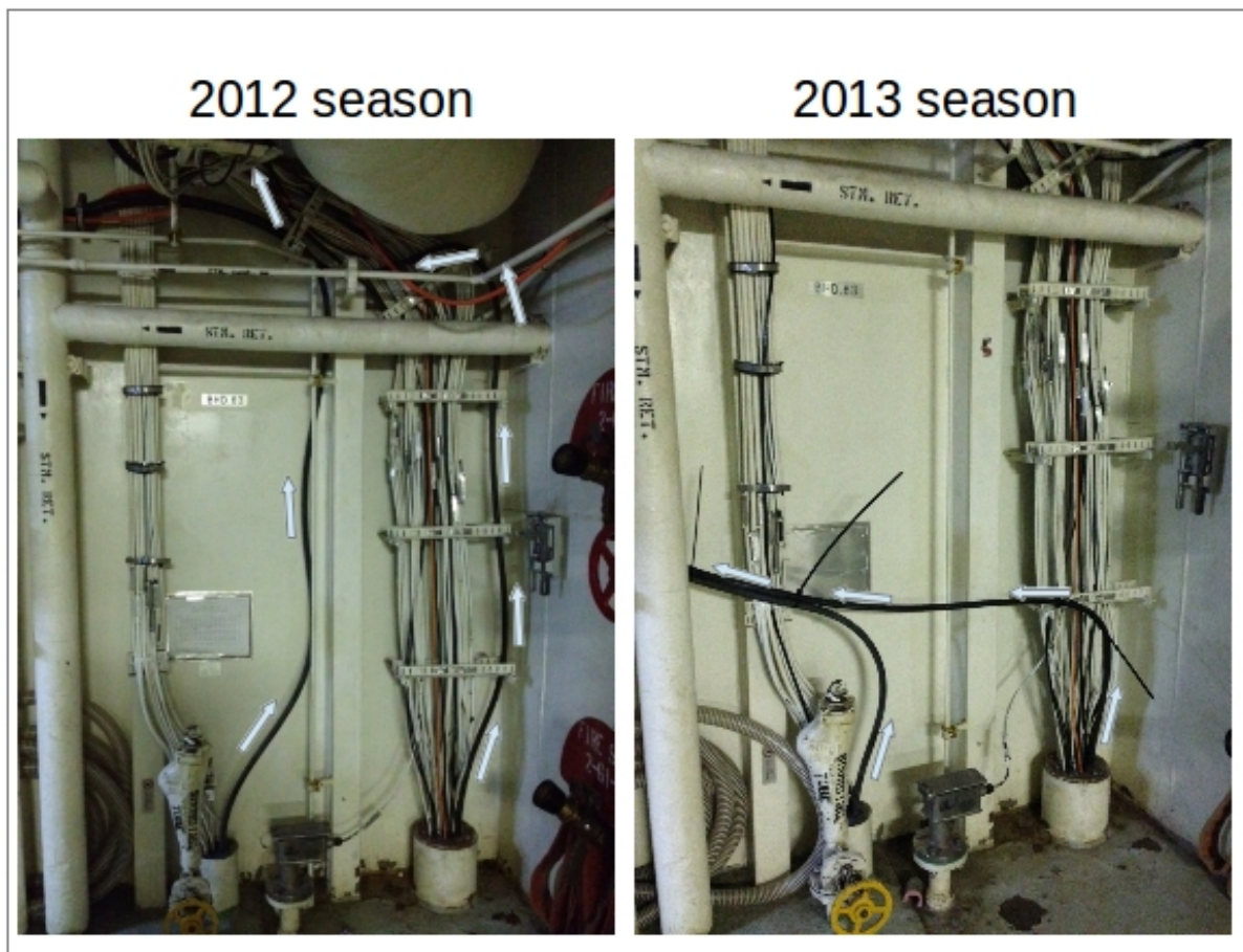
Figure 3: These photos show 'before' and 'after' positions of the cable near the through-hole from below the deck into MICA. The effect of this aspect of the transducer cable move was not investigated due to lack of time.
